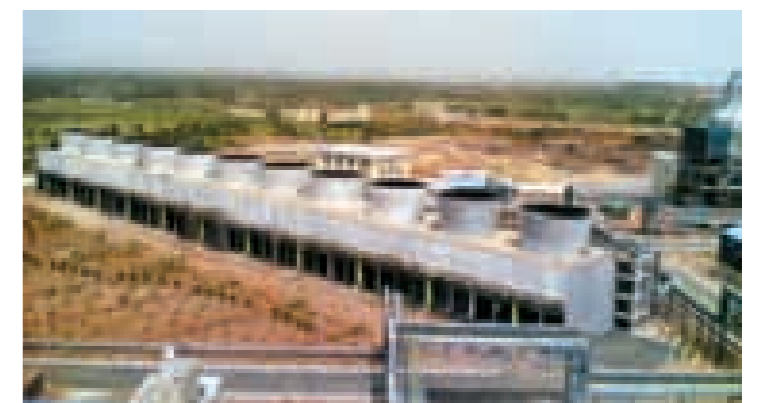
Induced draft cooling towers - part of L&T's comprehensive offerings to the power sector.
