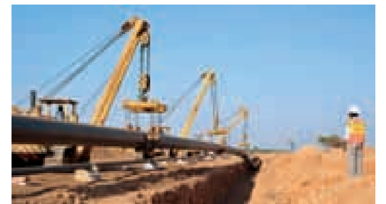
24" dia. x 592-km heated and PUF-insulated waxy crude oil pipeline being laid, along with an 8" gas pipeline.
