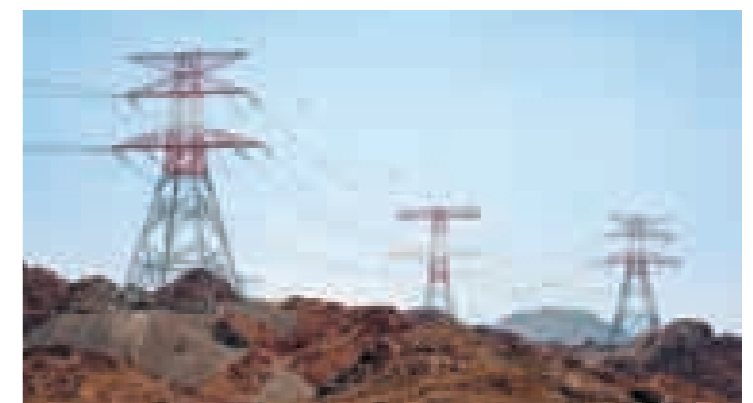
400 kV tranmission line projects executed by L&T at Fujirah-Dhaid, UAE.
